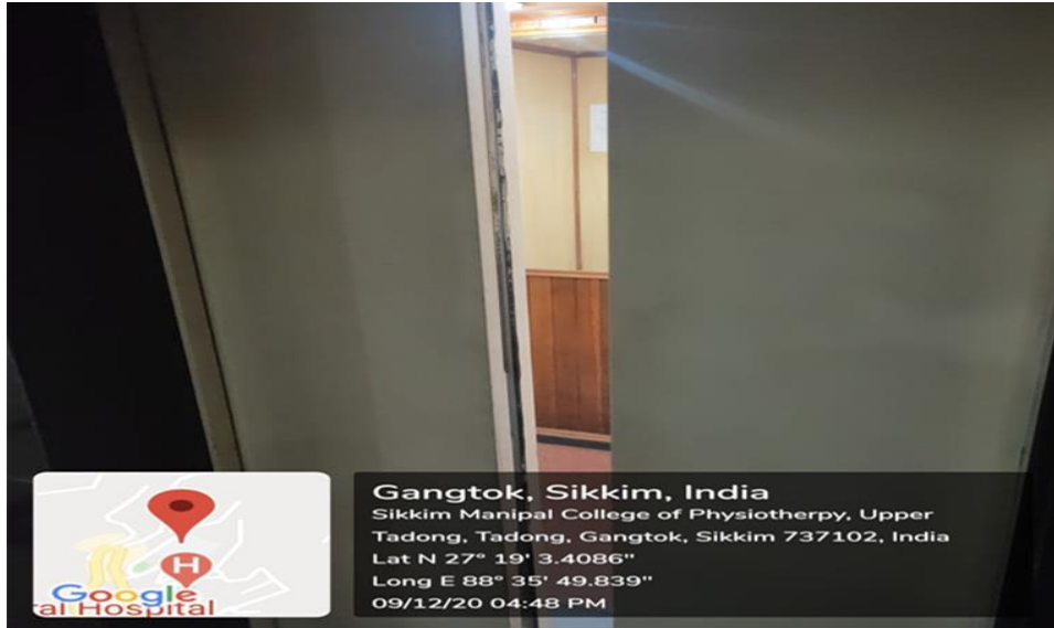
Automatic Doors in sensor-based escalators
