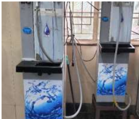
Water Cooler installed at campus
