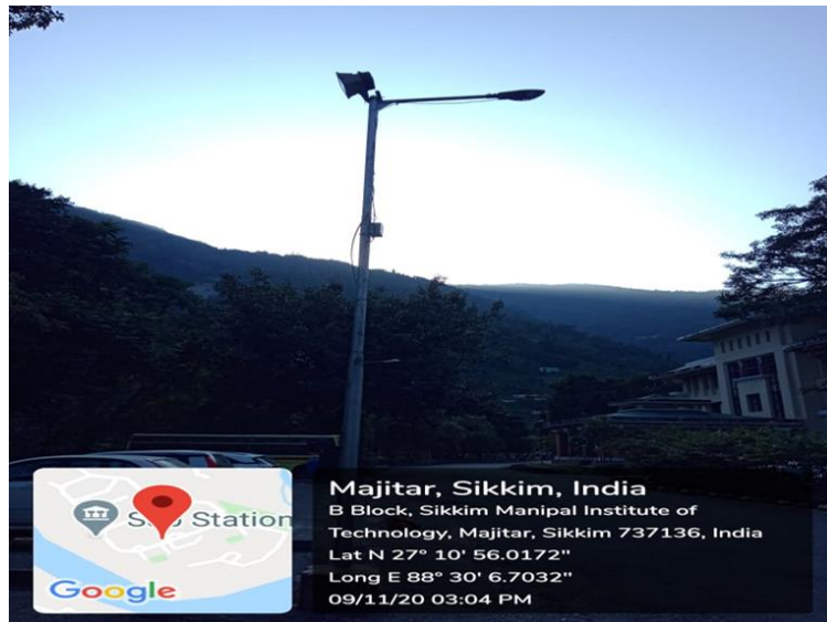
Sensor-based street light system at engineering campus
