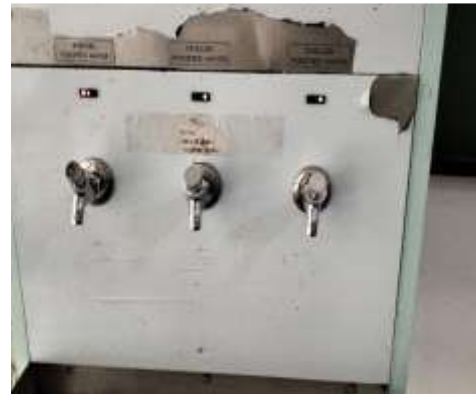
Push taps installed in water coolers
