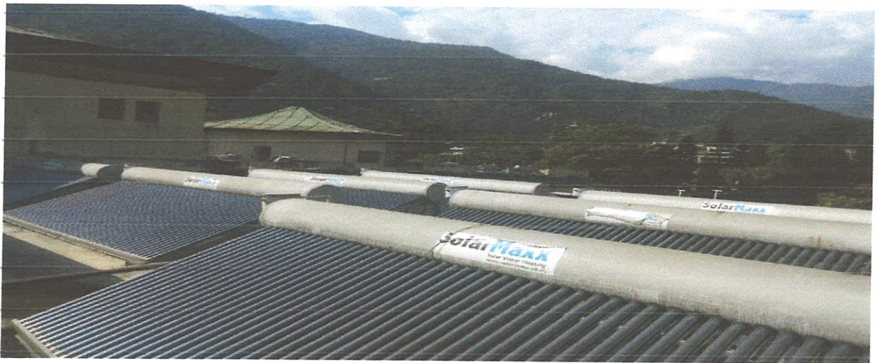
SOLAR WATER HEATERS AT SMIT CAMPUS
