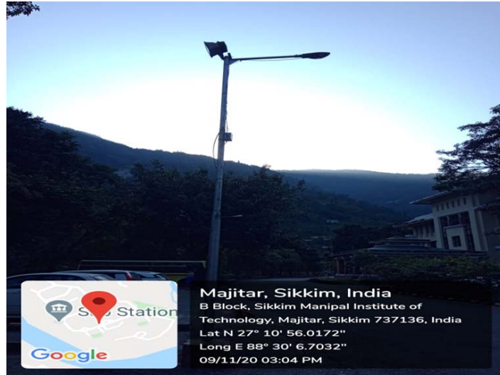
Sensor-based street light system at engineering campus
