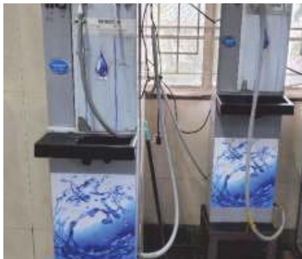
Water Cooler installed at campus
