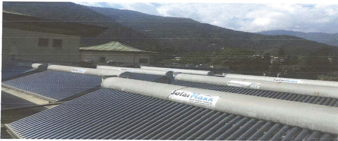
SOLAR WATER HEATERS AT SMIT CAMPUS
