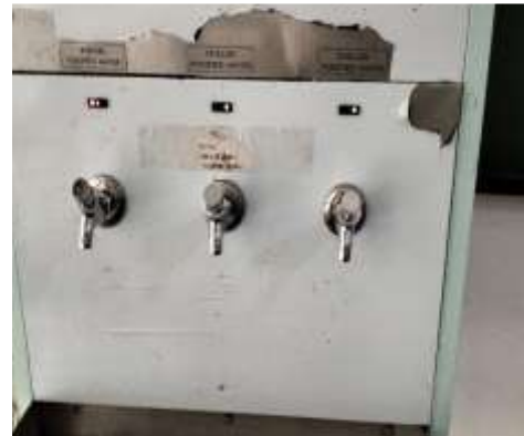
Push taps installed in water coolers
